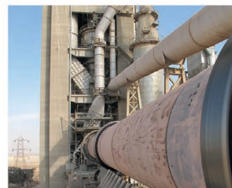
Beni Suef - Titan/Beni Suef Cement Co (Egypt) 4,000 tpd with 50% Alkali by-pass Gas or fuel oil
