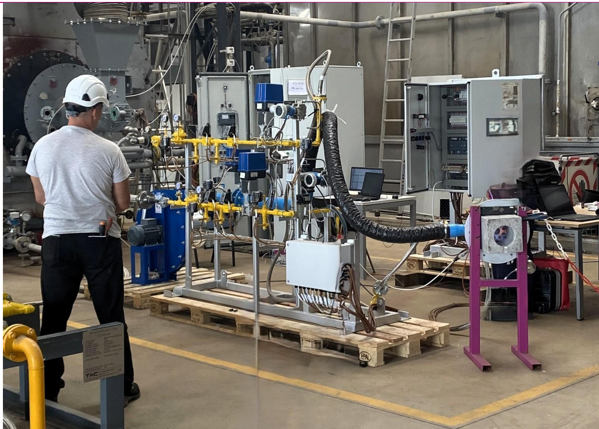
©Fives: Fives' hydrogen/natural gas burner tested and validated by Toyota
