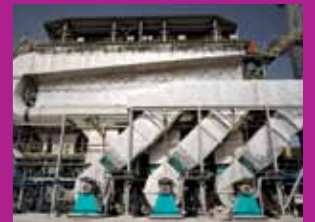
Page 34 • Partial view of a fume treatment center on an anode baking furnace
