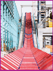
Page 6 • Partial view of a green anode plant under construction, dedicated to aluminium production
