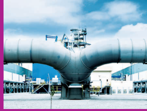
Page 8 • Gas treatment center, aluminium plant
