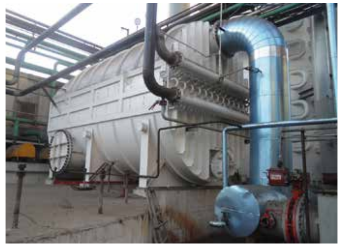
Reheater 1,400m 2 - Guatemala
